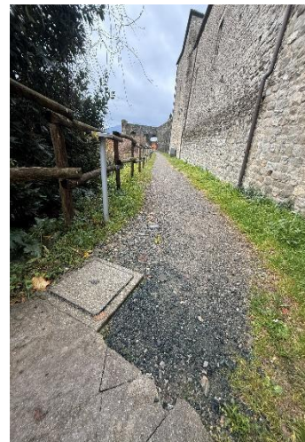
11 uneven and gravel pavement
